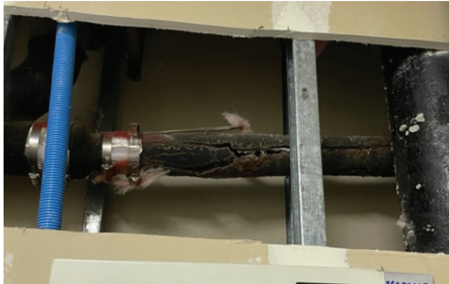
A recent photo of one of HPP's cracked drain pipes resulting in a water leak.
