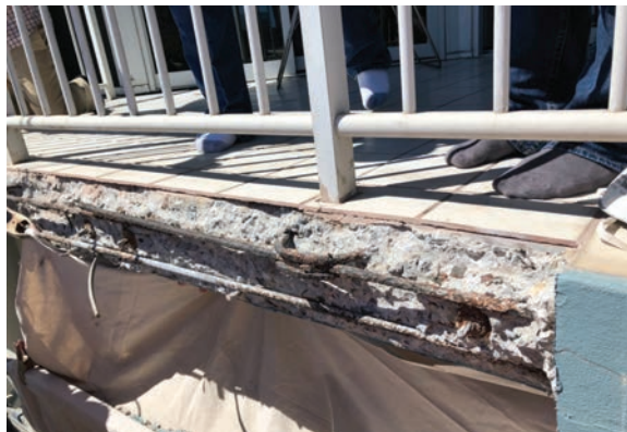
A damaged lanai at Honolulu Park Place
